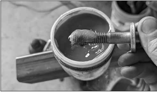
Dip the threads of the bolt in anti-spatter dip before assembling the bolt through the leg and positioning the nut
